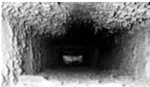
Before duct cleaning
