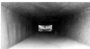
After duct cleaning
